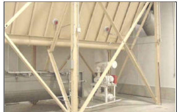
Installed Tender Blend Cooler (fig. 1) and Product Collector (fig. 2)
